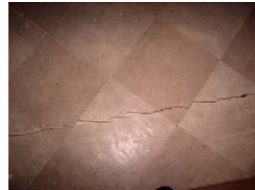
Fig.3 fissure de carrelage
