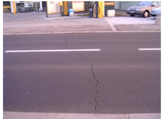
Fissure chaussée RN83 - Baume-les-Dames (Photo DDE)
